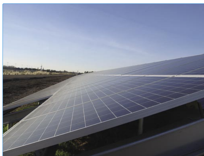
The solar panel array is capable of generating 756 Kilo Watts (KW) of electricity when the sun is ‘just right’.
