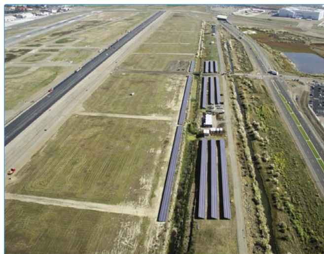
The zero emission solar energy system built on Port of Oakland property.
