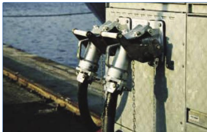
Figure 3. Shoreside electrical plugs.
