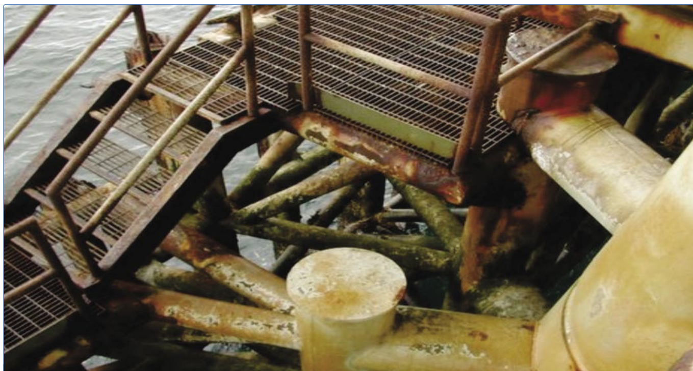
Salt water corrosion of boarding area on offshore platform.
