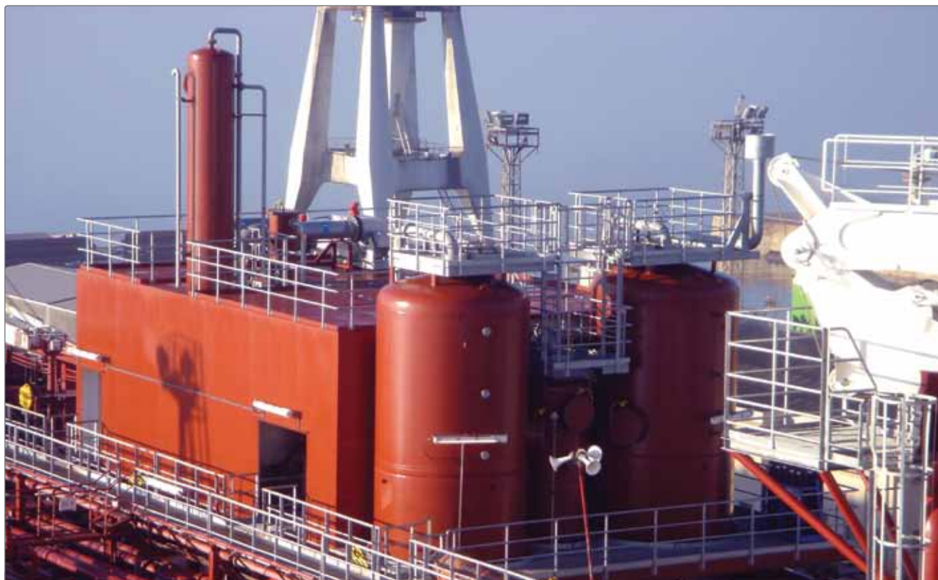
Åsgard C is installed aboard MIT Jorunn Knutsen operational in the Åsgard C field, North Sea.
