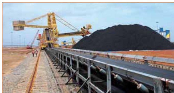
Yard conveyor with stacker-reclaimer.
