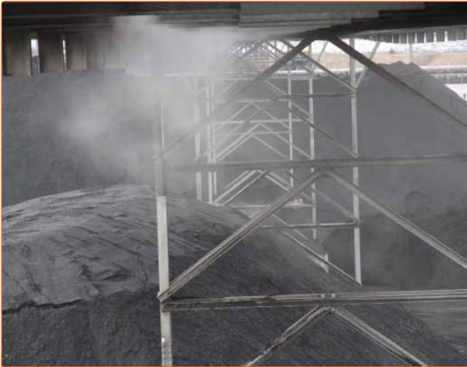
Fogging a tripper conveyor discharge.
