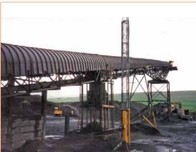
Covers fitted directly onto a conveyor.
